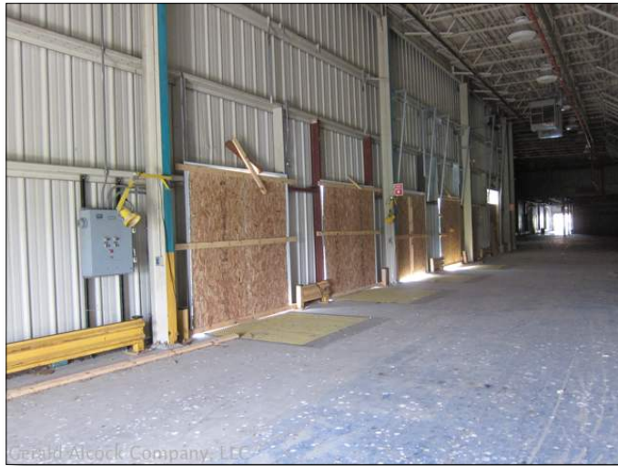
Shop Interior (Missing Overhead Doors)
