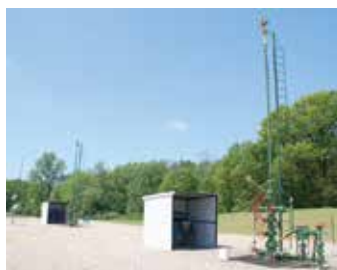
A wellhead at the Napoleon Field in Jackson County.
